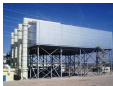
Hermosillo Sonora, Mexico — ACC for 350 MW Combined Cycle Power Plant
