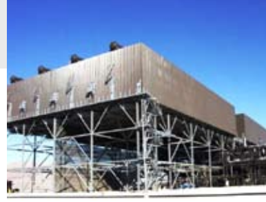
Big Horn Nevada, USA — ACC for 500 MW Combined Cycle Power Plant
