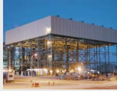
Apex Nevada, USA — ACC for 500 MW Combined Cycle Power Plant
