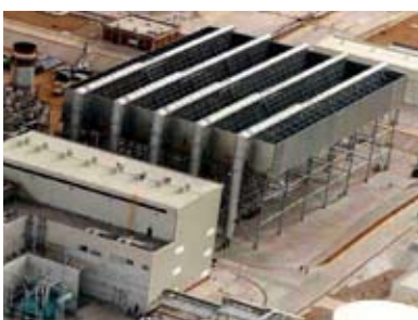
Chihuahua Chihuahua, Mexico — ACC for 450 MW Combined Cycle Power Plant
