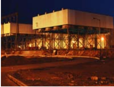
Monterrey Nuevo Leon, Mexico — ACC for 2 x 250 MW Combined Cycle Power Plant
