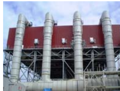
Astoria New York, USA — ACC for 500MW Combined Cycle Power Plant
