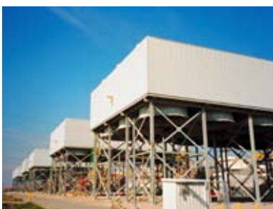
Midlothian Texas, USA — ACC for 6 x 250 Combined Cycle Power Plant
