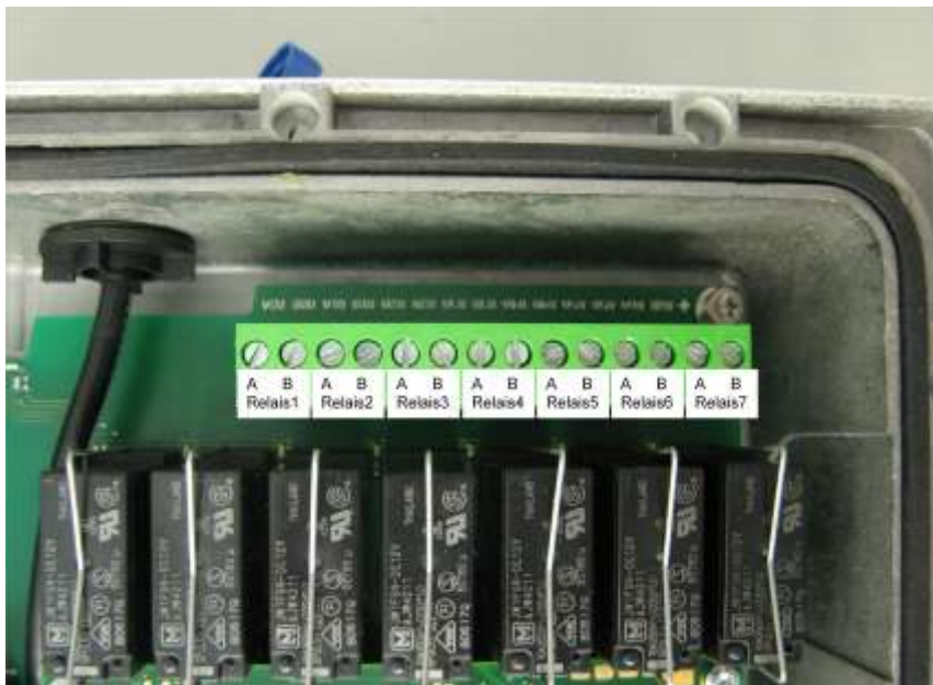
Figure 9: Relay terminal block B1
