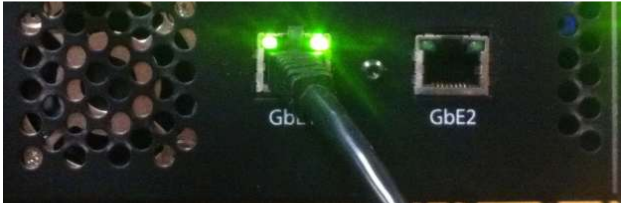
Figure 68 – Network Connectivity Indicator LEDs
