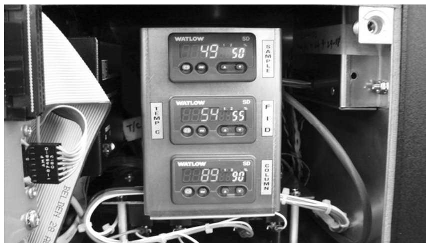
Figure 2-1: Internal Temperature Controllers
