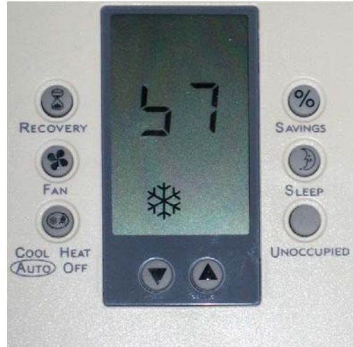
Figure 3 : Thermostat showing Signal Strength from Sensor
