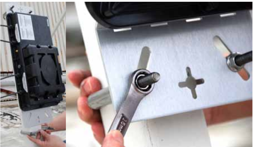
Figure 1. Showing mounting of SolarMagic powerstring optimizer to a PV array support tower.
