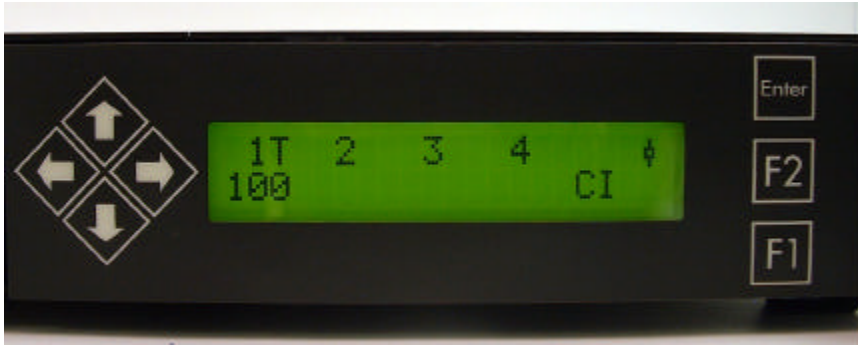
Figure 38 - Communication Integrity Status for a Wired Tracking Station 1
