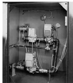
Factory assembled gas manifold compartment
