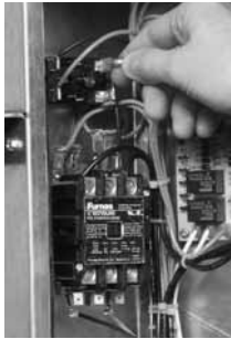
Figure 64. Connecting speed-tap wire
