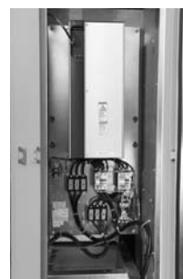
Figure 6. Variable frequency drive
