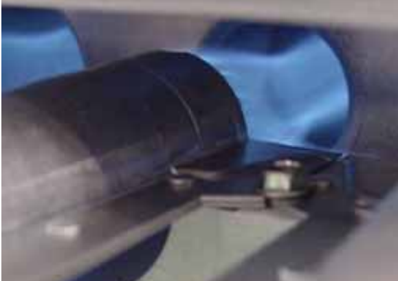
Burner flame at start-up: 1.2 in. wc manifold pressure draft inducer—high speed
