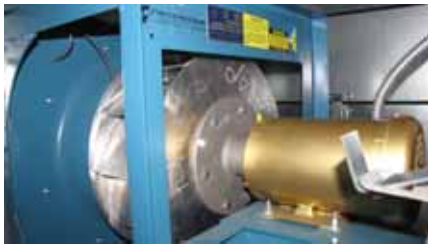
Figure 4. Plenum fans help reduce noise levels
