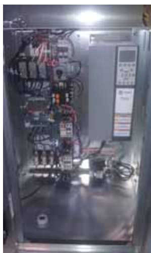
Figure 5. Integral controls cabinet for starters, variable frequency drives, and unit controllers
