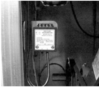
Figure 56. Piezometer ring measures inlet air flow.
