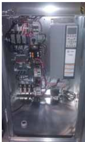
Figure 116. Internally mounted VFD
