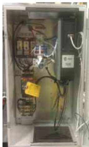
Figure 117. Externally mounted VFD
