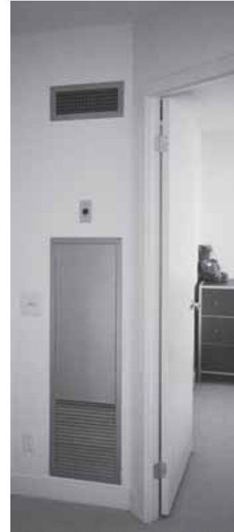
Figure 2. Furred-in fan coil
