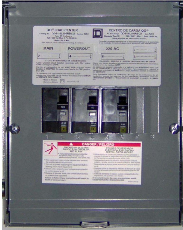
Figure 4-1 Breaker Panel 1 (with front cover raised)
