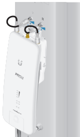
Connecting to a Sector Antenna
