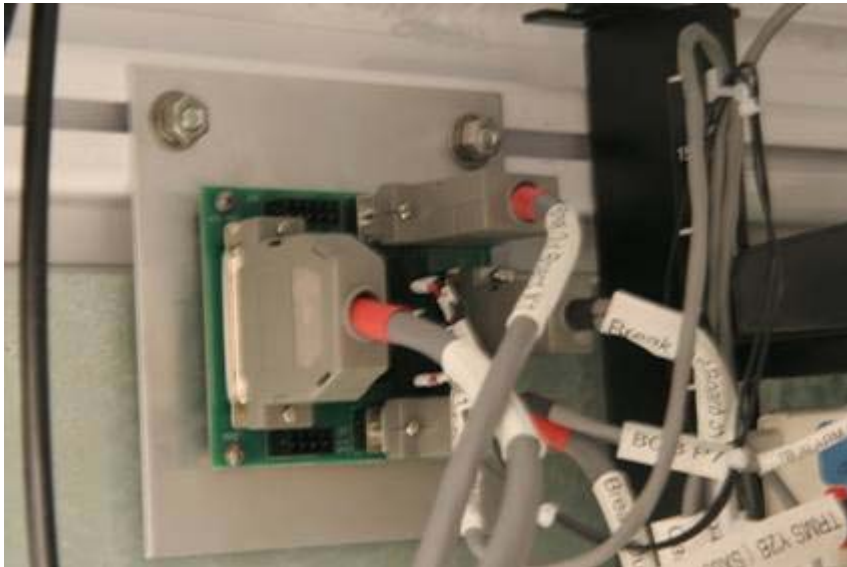
Figure 3-32 Break Out Board Installed in DRU
