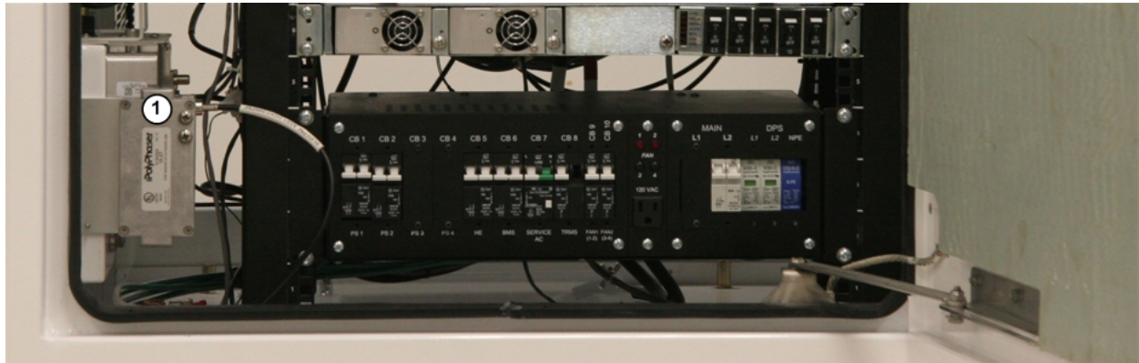
Figure 3-30 Telco Surge Protector
