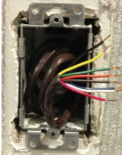
Fig. 2 -- Coil Excess Wiring
