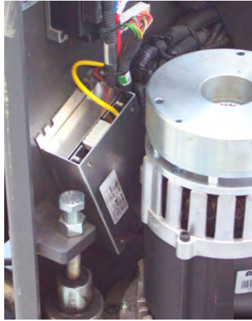
Figure 17: Power Supply Attached to a Secure Surface on the Vehicle
