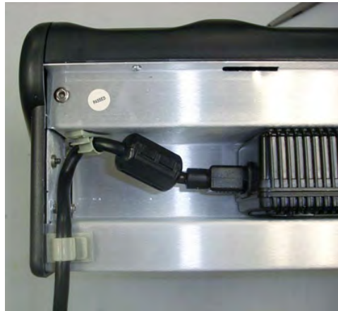
Figure 25: Cable Routed Through Plastic Clips
