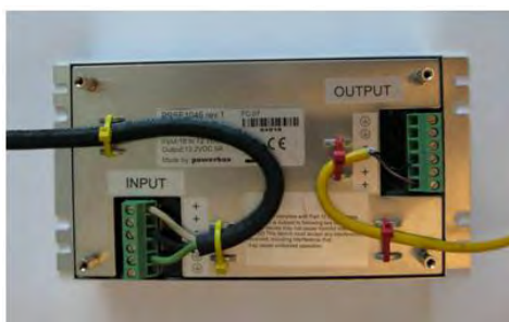
Figure 16: Cables Attached to the Power Supply
