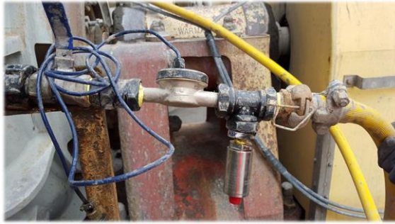
Figure 13-8 Gland water sensor installation
