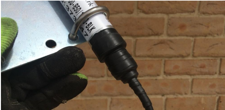
Figure 6-18 Antenna connector wrapped in protective tape
