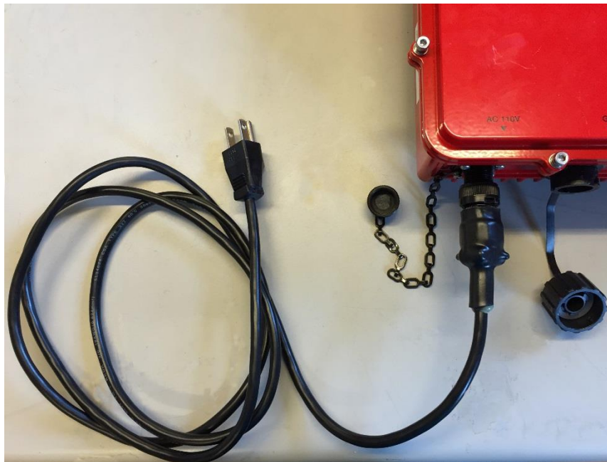
Figure 5-10: Power Cable Connected to Repeater
