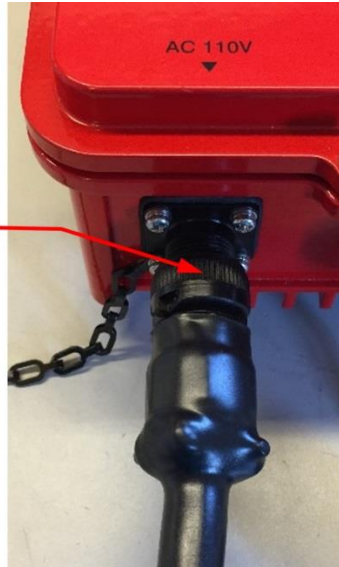
Figure 5-9: Power Cable Connected to Repeater
