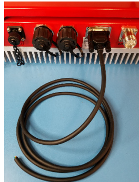
Figure 5-5: Alarm Relay Cable Connected to Signal Booster
