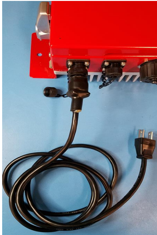
Figure 5-10: Power Cable Connected to Signal Booster
