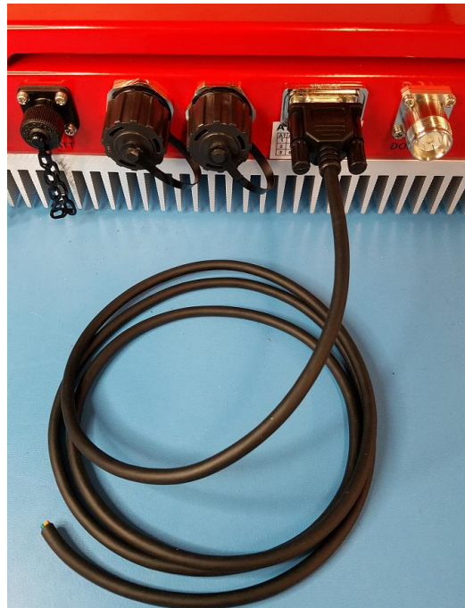
Figure 5-6: Alarm Relay Cable Connected to Signal Booster
