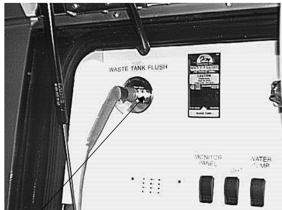
Flushing System Inlet
