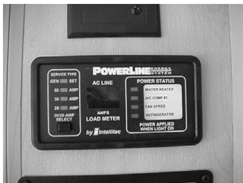
EMS System Panel
