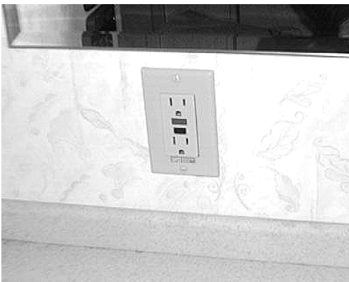
Ground Fault Circuit Interrupter (GFCI)
