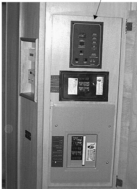
Monitor Panel - Model 36C Across Hall from Refrigerator
