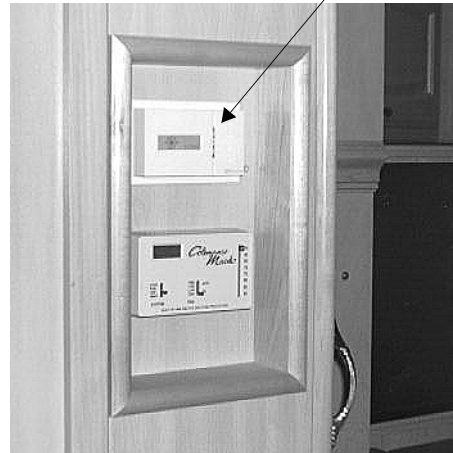
Power Ventilator Thermostat - Galley
