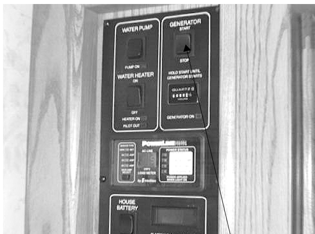
Generator Switch and Hourmeter
