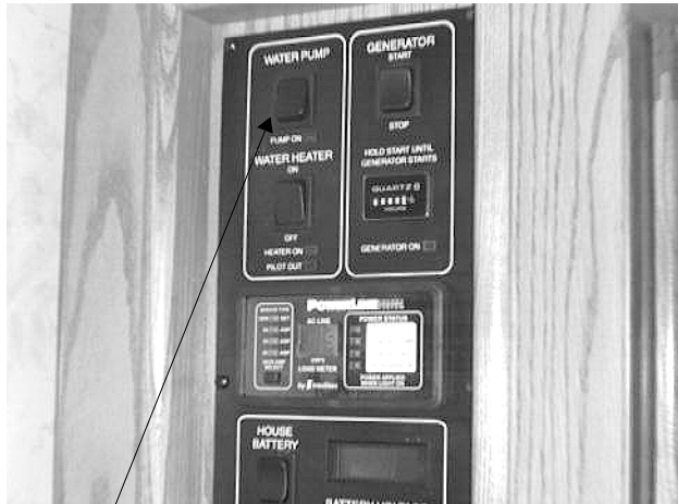
Water Pump Switch
