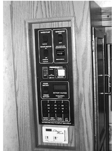
Monitor Panel - Model 38K In Hallway Across From Refrigerator
