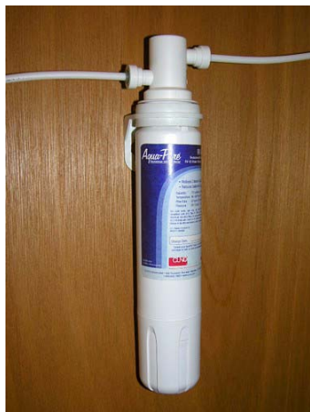
Water Filter Assembly below Galley Sink
