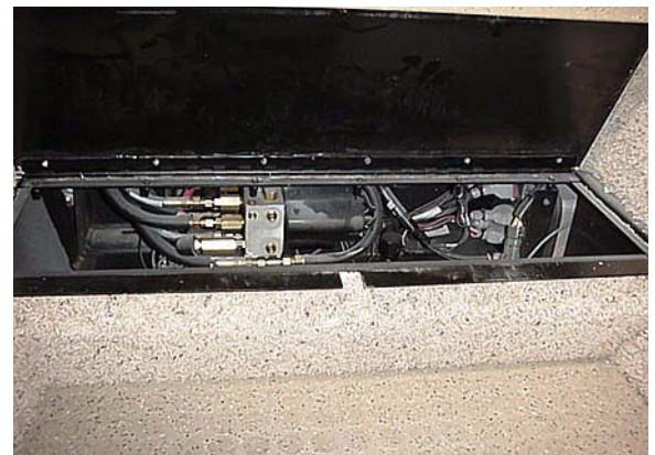
Hydraulic Pump beneath Entry Step
