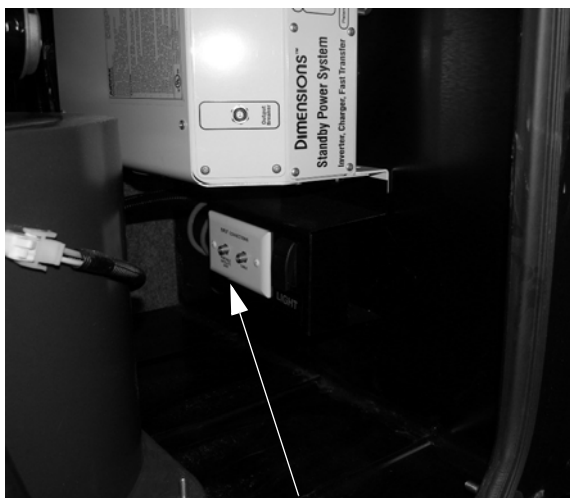
Exterior Input Connections for Satellite Dish and Cable TV (in Water Center or Utility Compartment)
