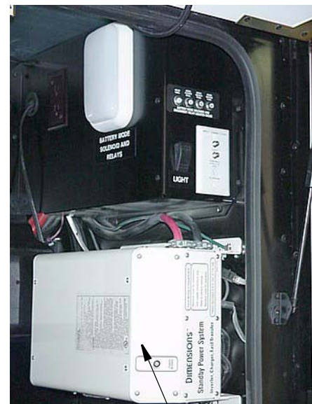
Inverter Charger Unit Location (in utility compartment)
