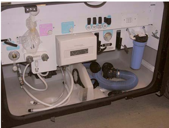
Water Service Center - Typical View
