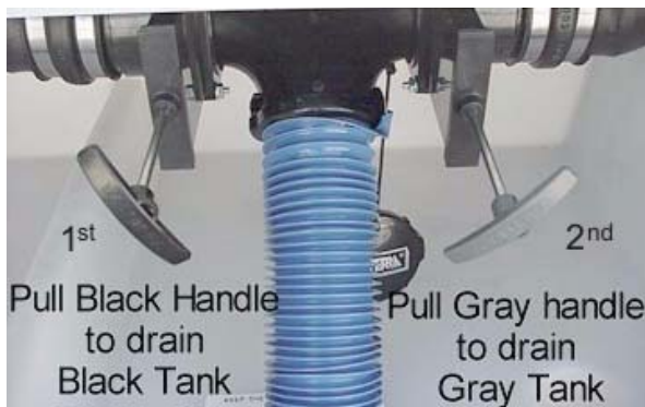
Holding Tank Valves (Typical)
