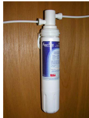
Water Filter Assembly below Galley Sink
