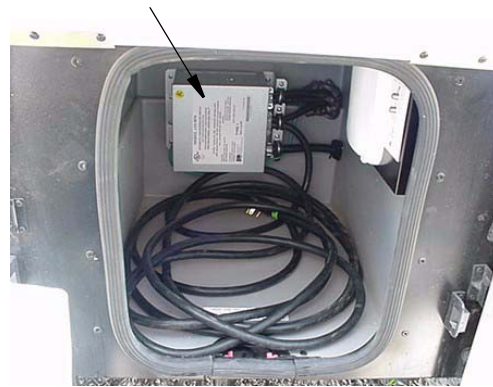
Power Transfer Switch
