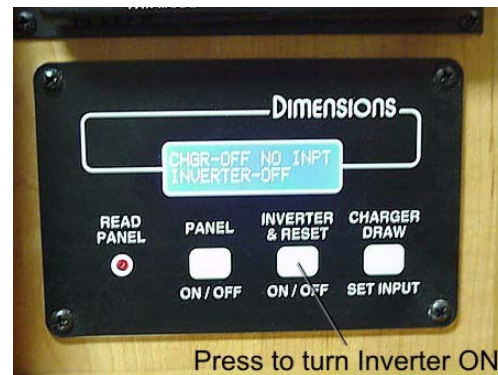
Inverter/Charger Control Panel
