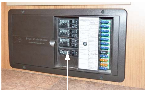
120-Volt Circuit Breakers -Typical View
