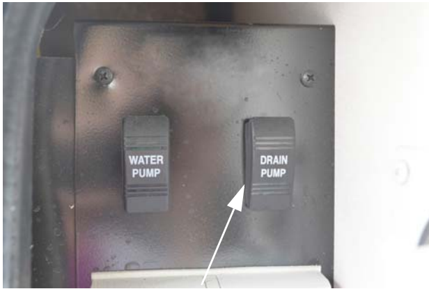
Waste Pump Switch (Located in water service center)
