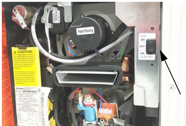
Water Heater Mode Switch (Located behind water heater access panel on exterior of coach)
