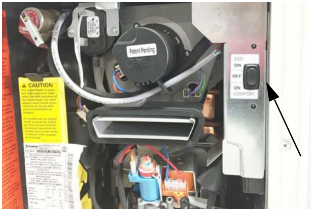
Water Heater Power Switch (Located behind water heater access panel on exterior of coach)
