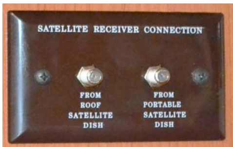
Interior Connection for Satellite Dish (Located near entertainment center cabinet) -Typical View
