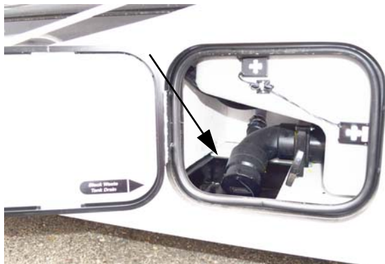
Sewage Drain Outlet (Located in driver side compartment ahead of rear wheel)
