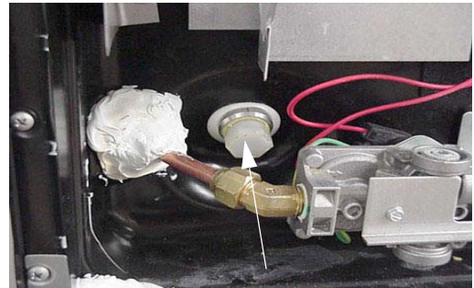
Water Heater Drain Plug (Remove with socket)
