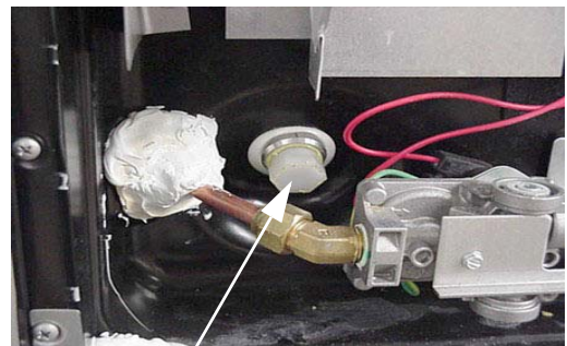
Water Heater Drain Plug (Remove with socket)
