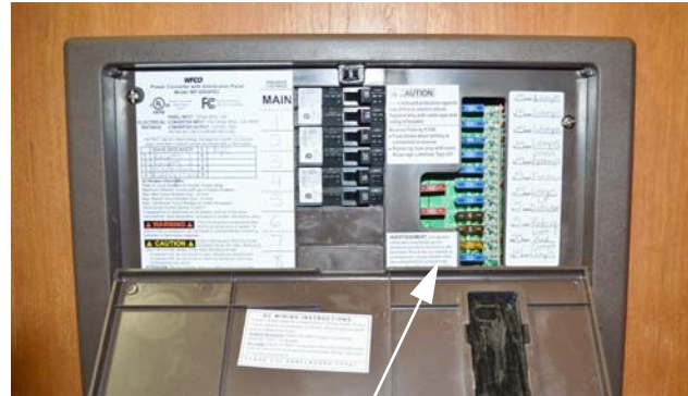
House 12-Volt Fuses (Located on the right-hand side of the power converter) -Typical View
