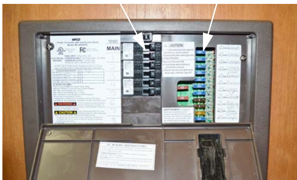
Power Center (Converter) -Typical View
