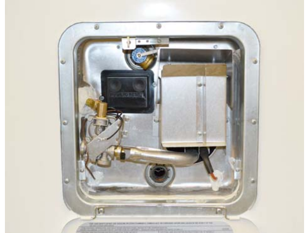
Water Heater Exterior Service Access
