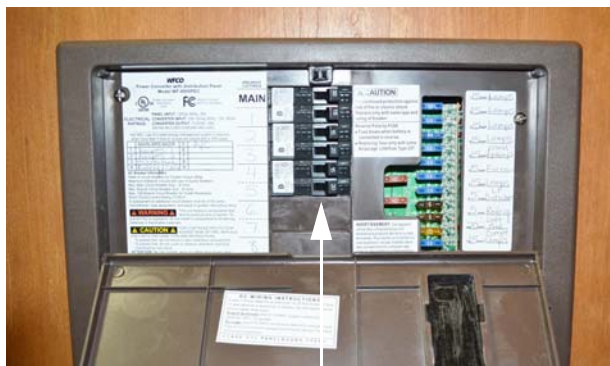
120-Volt Circuit Breakers -Typical View
