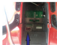
The port inside the battery box.
