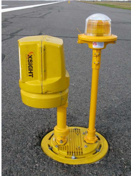
Figure 2: Sensor installed next to an edge light
