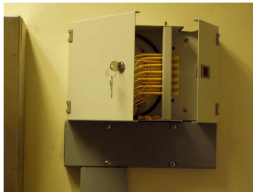
Figure 9: Field patch panel
