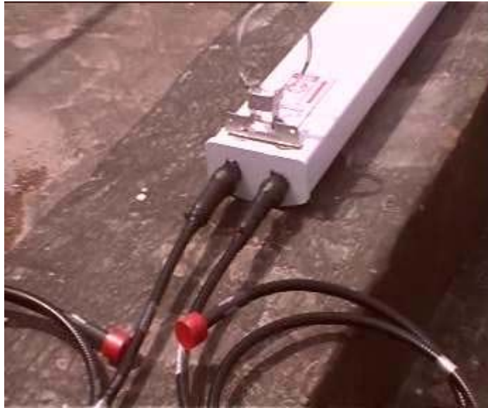
FIGURE 72 CONNECTION BETWEEN DIRECTIONAL ANTENNA AND JUMPER
