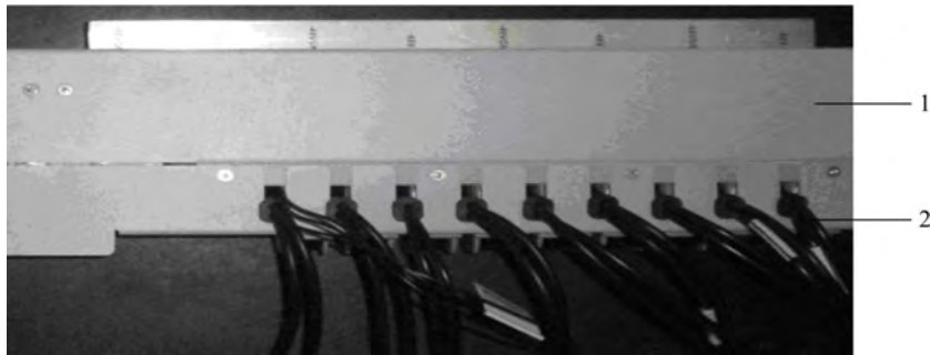
Figure G-5 BBU and RRU Power Cable Installation
