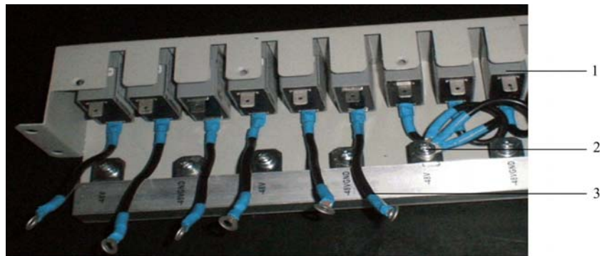
FIGURE 152 INSIDE CABLE TO CONNECT WITH PDM
