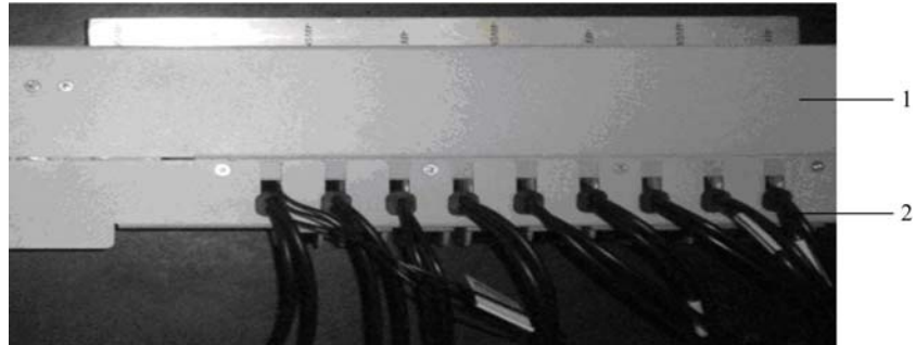
FIGURE 154 BBU AND RRU POWER CABLE INSTALLATION
