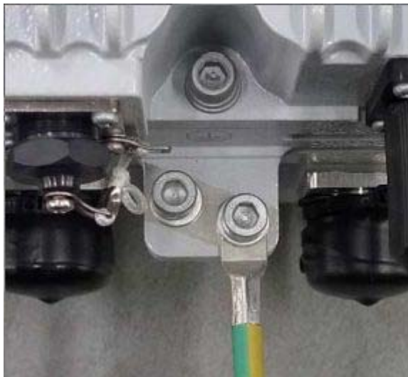
Figure 3-40 R8882 Grounding Bar Connection
