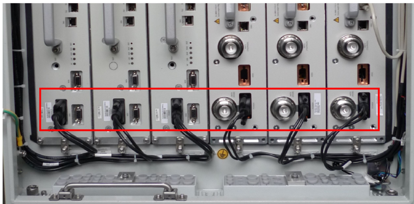
Figure 5-8 Power Cable Connecting the RSU
