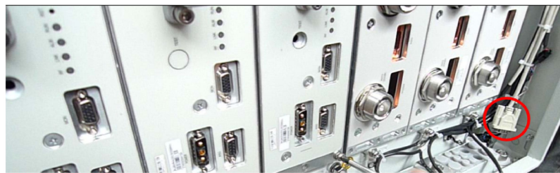
FIGURE 13 RSU MONITORING CABLE
