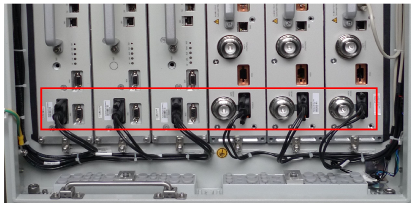
FIGURE 12 POWER CABLE CONNECTING THE RSU
