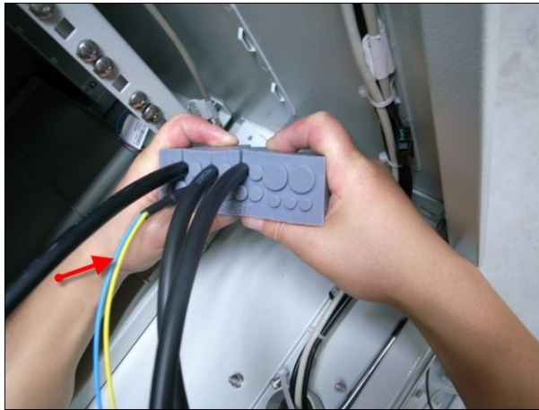
Figure 5-11 Waterproof Module through Which Optical Fibers Pass
