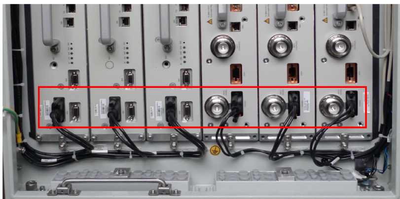
Figure 5-8 Power Cable Connecting the RSU
