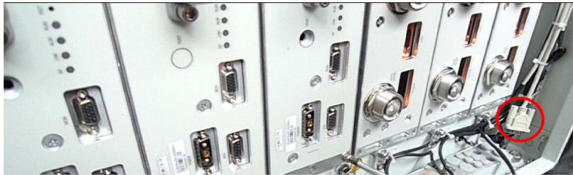
Figure 5-9 RSU Monitoring Cable
