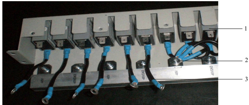
FIGURE 143 INSIDE CABLE TO CONNECT WITH PDM
