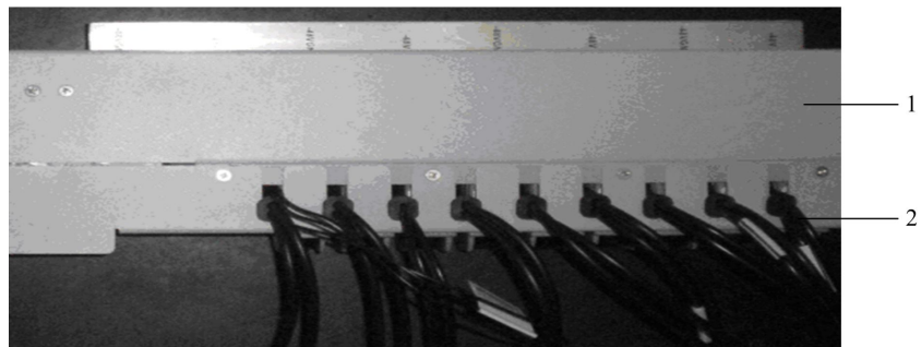
FIGURE 145 BBU AND RRU POWER CABLE INSTALLATION
