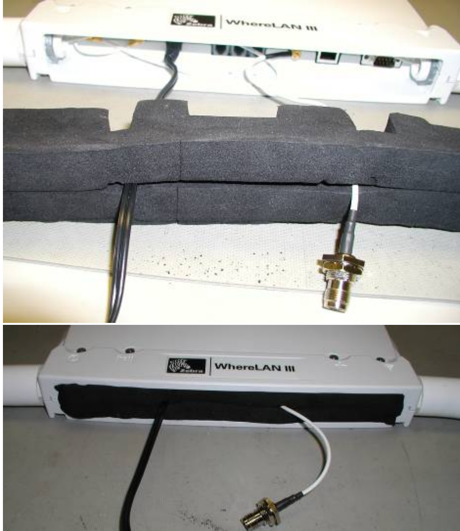
Figure 26 Wi-Fi Cables Drip Plug
