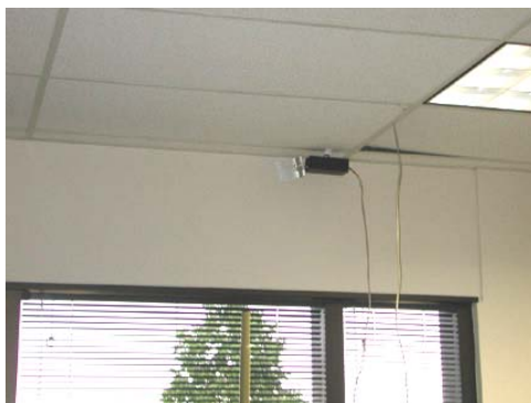
Figure 2. Another typical ceiling mount for PAL-650 Receiver.
