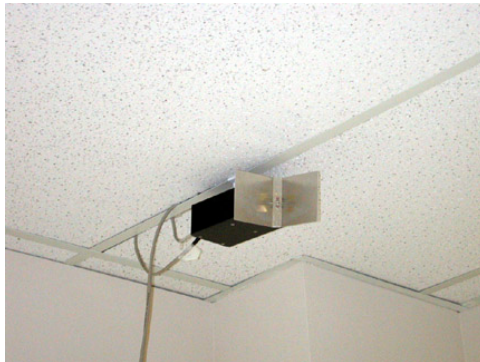
Figure 1. Typical ceiling mount for PAL-650 Receiver. Note placement of directional antenna (pointing inwards).
