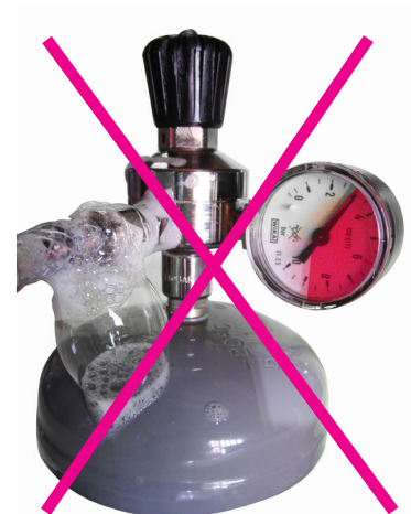
Faulty seal joint
