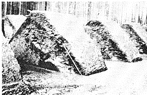
Fig. 2—Pitting in concrete baffles in the Bonneville Dam stilling basin after 17 years of heavy service.
