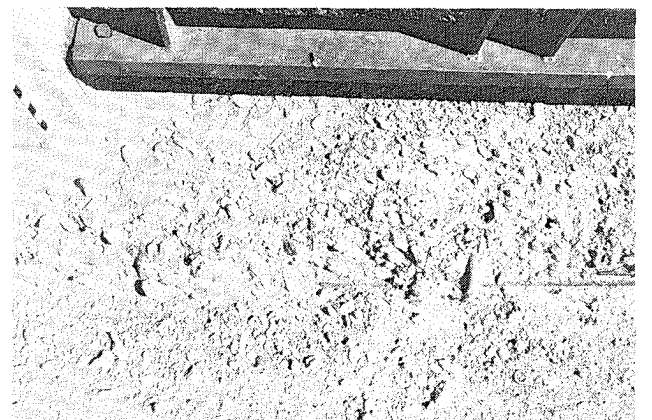
Fig. A.2.9.5.b—Close-up of scaling (very severe)
