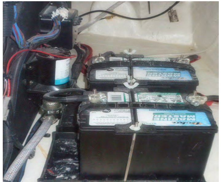
TYPICAL MAINTENANCE FREE BATTERIES
