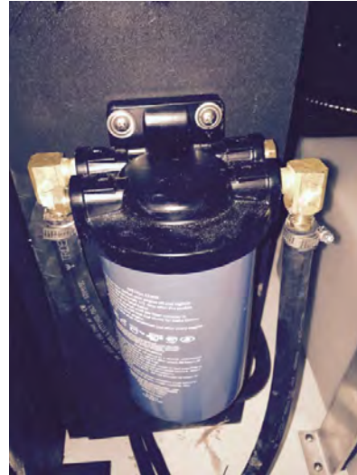
CHECKING IN-LINE WATER SEPARATOR FILTER
