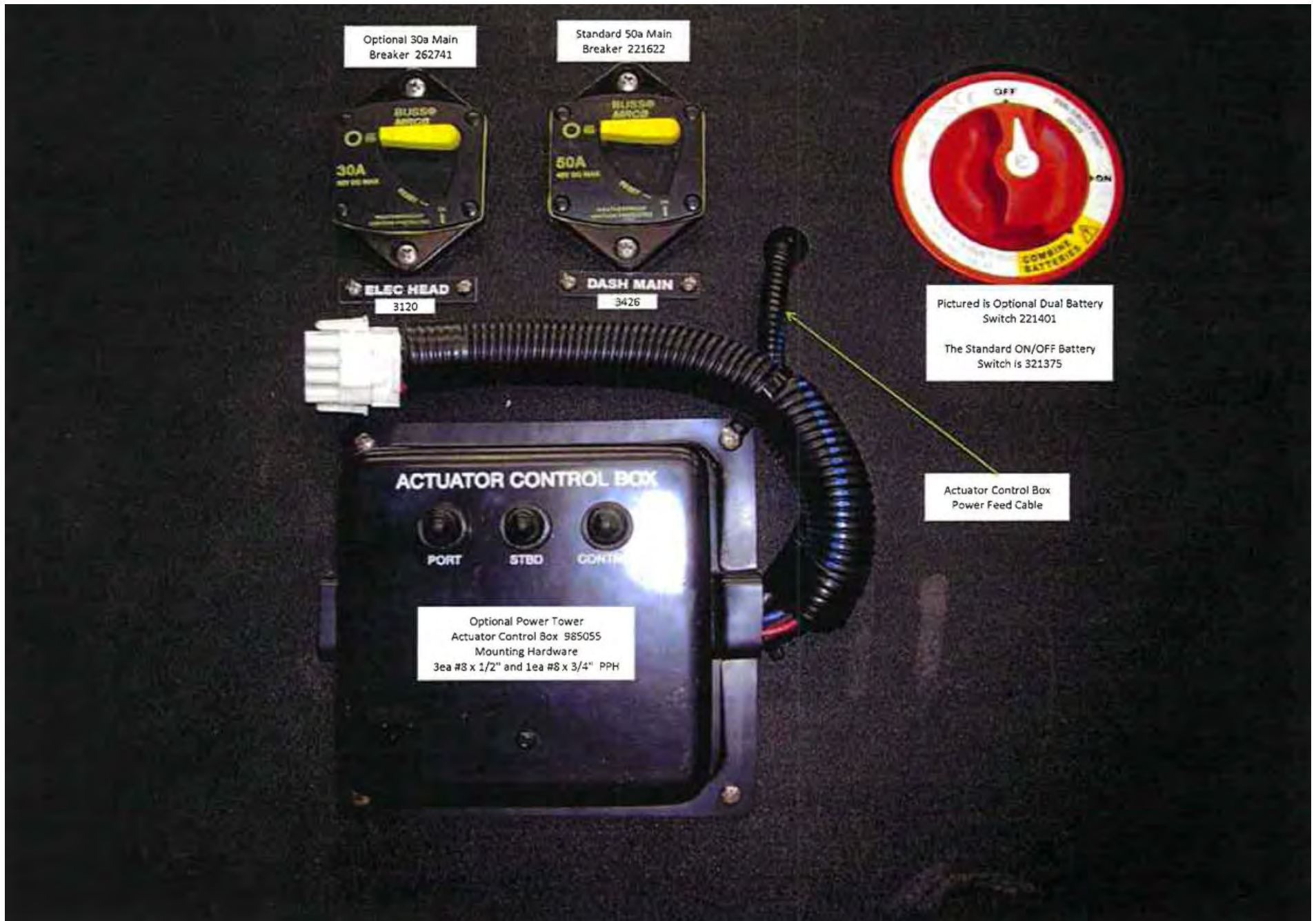
26 FASDECK BATTERY MANAGEMENT PANEL
