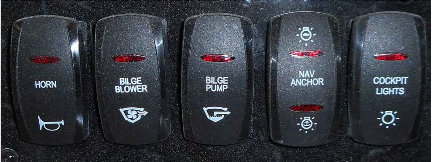
PORT SWITCH PANEL
