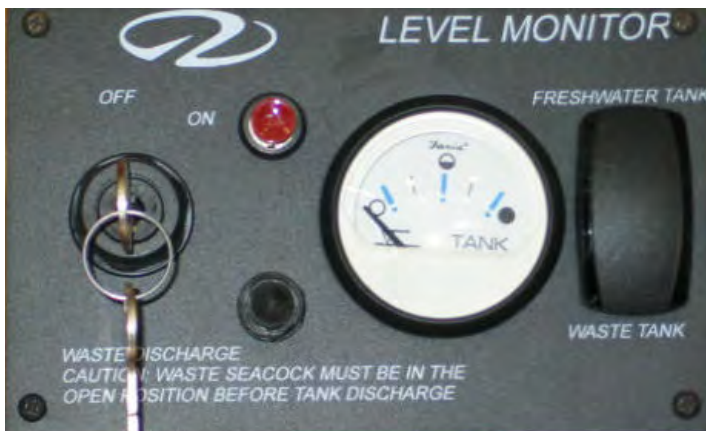
TYPICAL WATER/WASTE MONITOR PANEL
