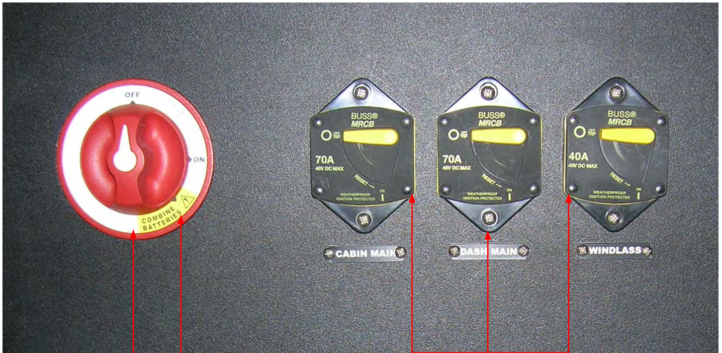
ENGINE BATTERY SWITCH
