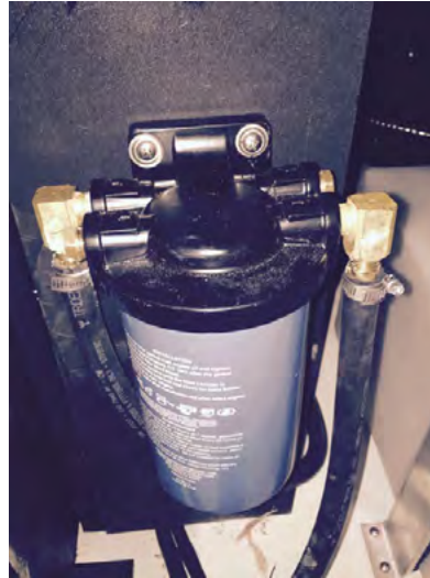
CHECKING IN-LINE WATER SEPARATOR FILTER
