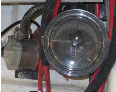
TYPICAL A/C SEAWATER STRAINER/BASKET
