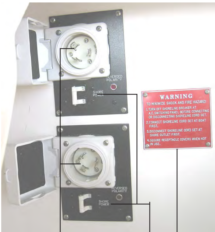
TYPICAL SHORE POWER INLETS
