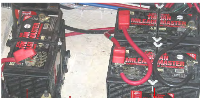
PORT ENGINE CRANKING BATTERY
