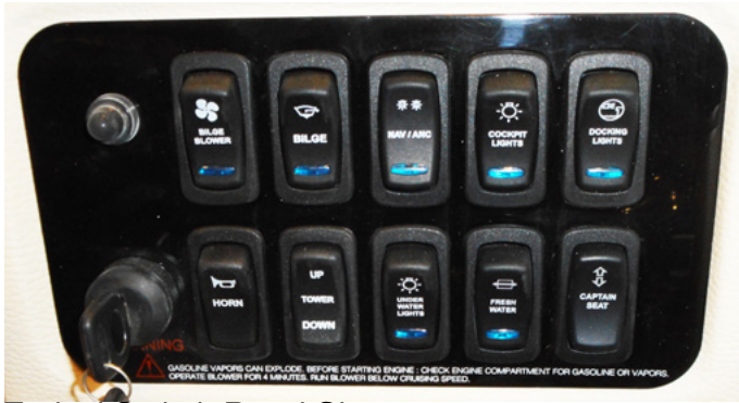
Typical Switch Panel Shown
