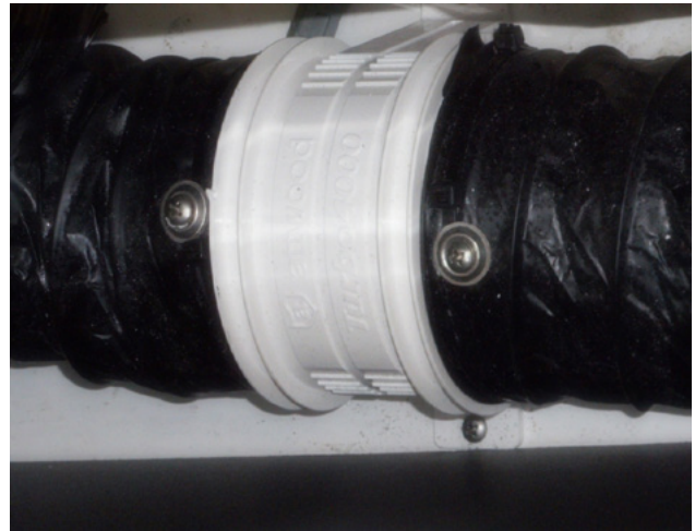
Typical Ventilation Blower with Hose
