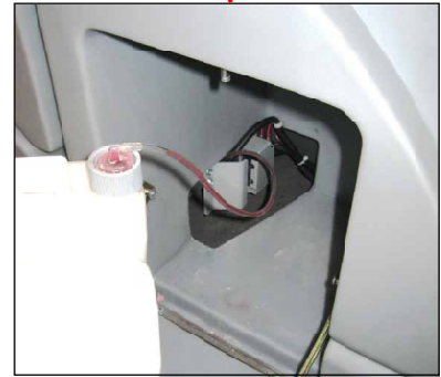
AXP Pumps (behind cover panel)
