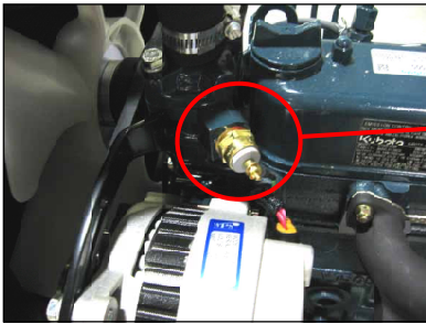
Coolant Temperature Sensor (above alternator)
