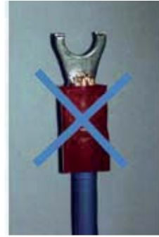
Terminal has been cut.
